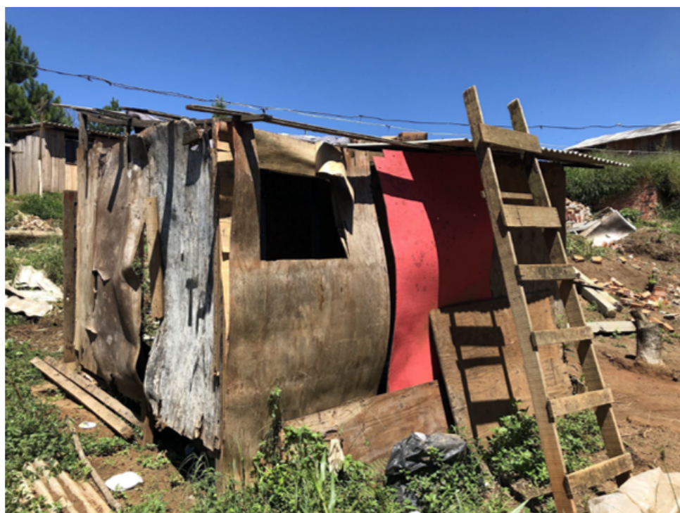
Figure 1 – Typical Control Housing Unit
